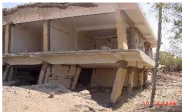
FIGURE 2: RC BUILDING IN BHACHAU COLLAPSED DUE TO SWAY MECHANISM
